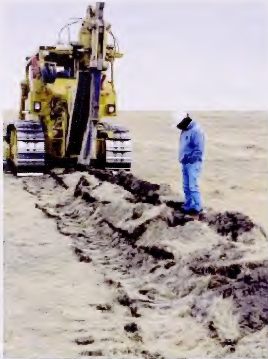
Photo 15 The type of equipment used must be appropriate for the soils and the timing of construction.
